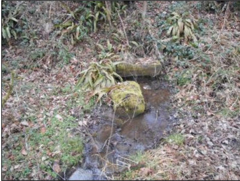
Water from road to toe area.
