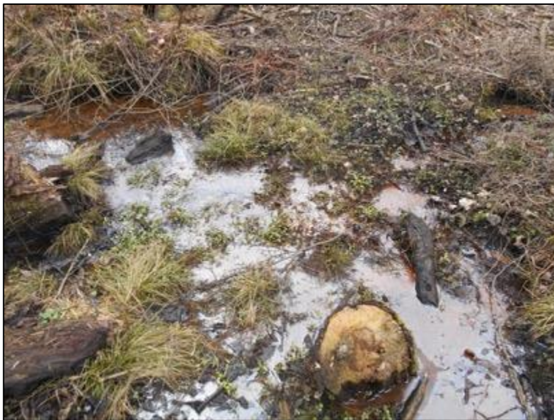
Downstream toe area – no drainage due to absence of gradient away from dam toe.
